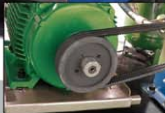
3 Phase, 18 – 22 amp, 15 Hp Motor
